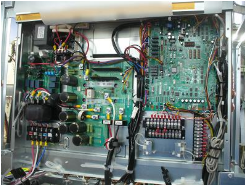
Air to water unit
